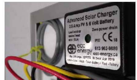
Figure 9 Solar panel battery charger
